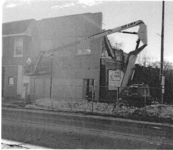
Demolition crews took down the blighted commercial structure at 1806 Sheridan Road on February 3, 2021.
